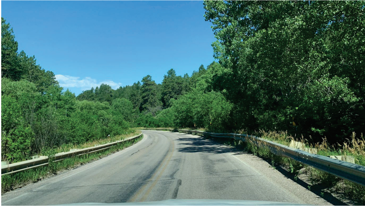
Figure 26: Existing Damaged Guardrail, Excessive Vegetation Covering Signage and Narrow BIA 4 Roadway
