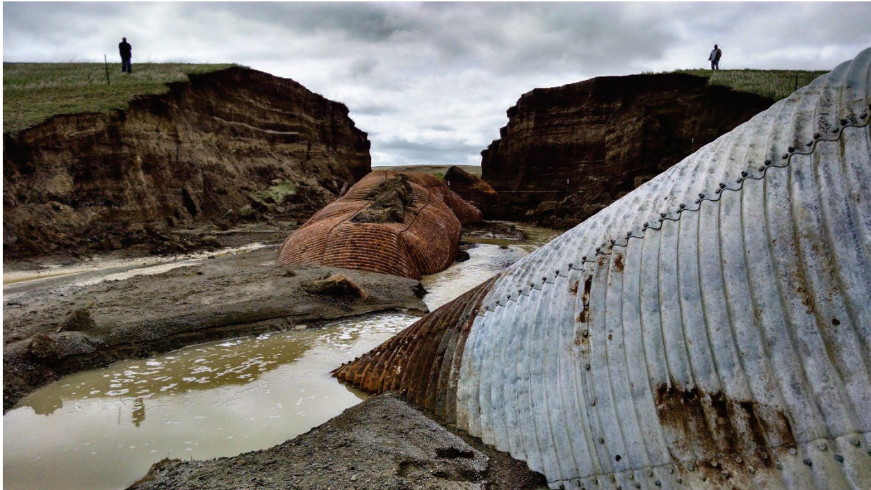
Figure 21: Culvert Failure Along BIA 2
