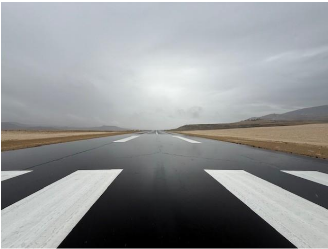
Figure 2-6 – Condition of Runway 11/29
